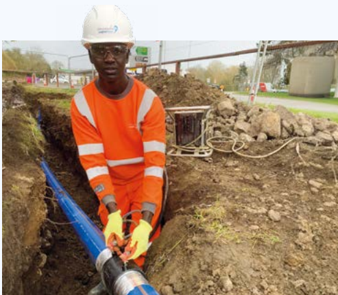
The Collaborative Skills Programme sponsors full-time courses in Construction and Engineering at four colleges across our region – Yasser Osman, an apprentice groundworker hard at work welding water pipe with electrofusion box.
